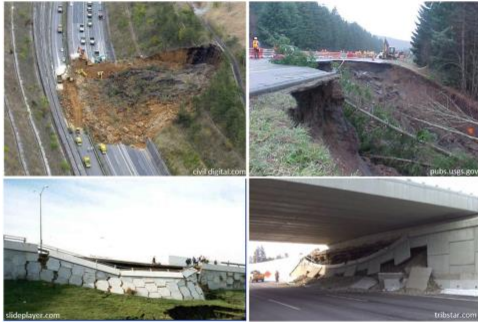
Figure 1. Failure examples affecting traffic corridors
