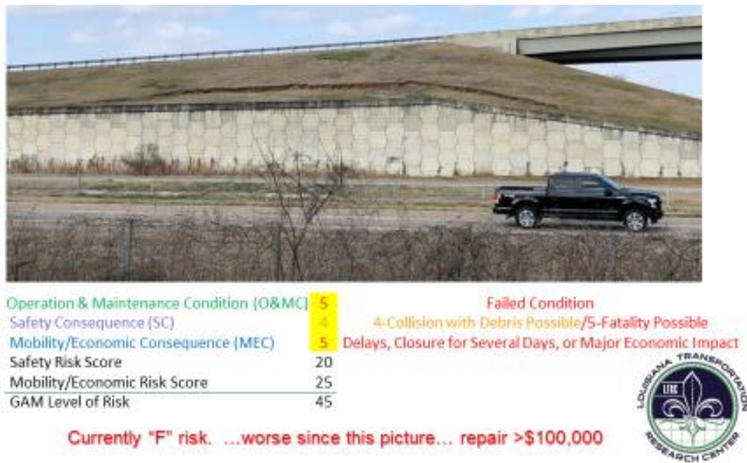
Figure 38. Example rating and LOR, I-49 ramp to LA 3132 West, Shreveport, LA
