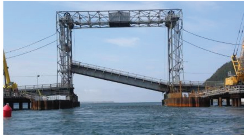
Figure 1. A vertical lift bridge rendered non-functional due to a severely skewed deck
