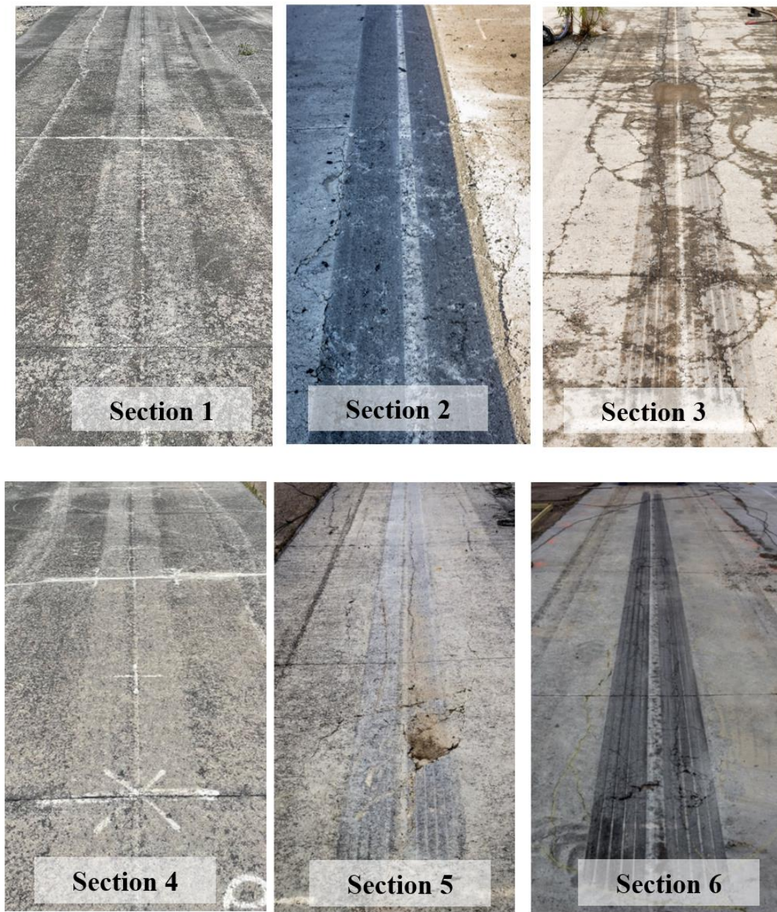
Figure 19. RCC pavement condition at the end of testing
