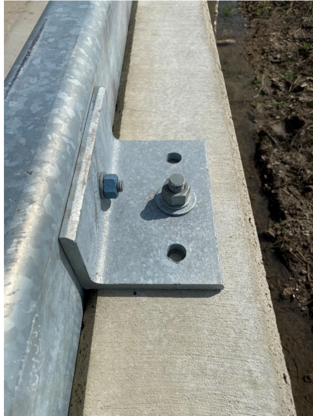
Figure 94. Installed L6×4×½ angle support bracket with ¾-in. A193 B7 galvanized threaded rod with Hilti RE500-V3 adhesive
