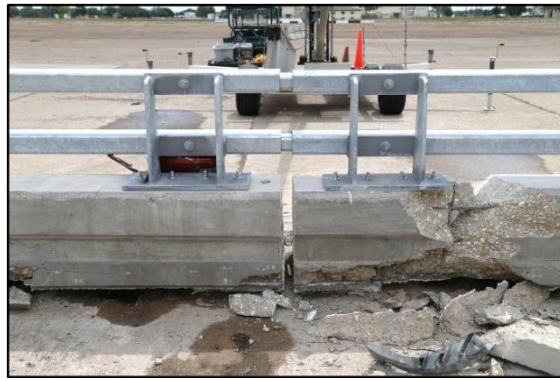
(b) Field side damage
