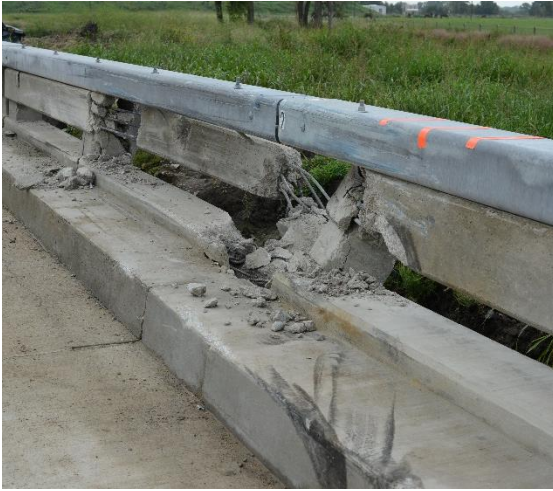
(a) Damage to curb and beam
