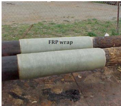
Figure 17. Electrical poles with FRP wraps
