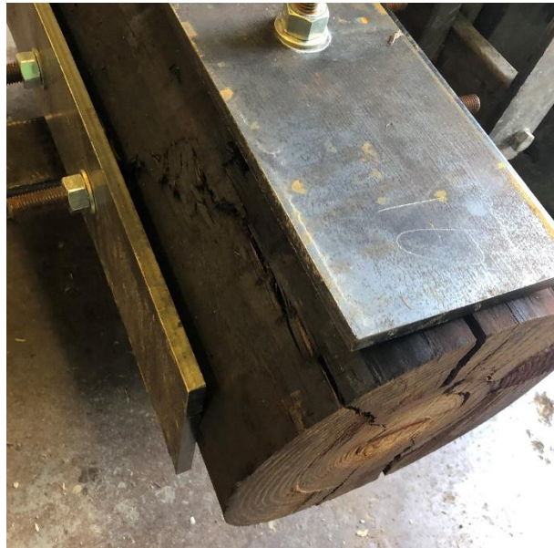
Figure 121. Buckling near contact surface of steel splice pile
