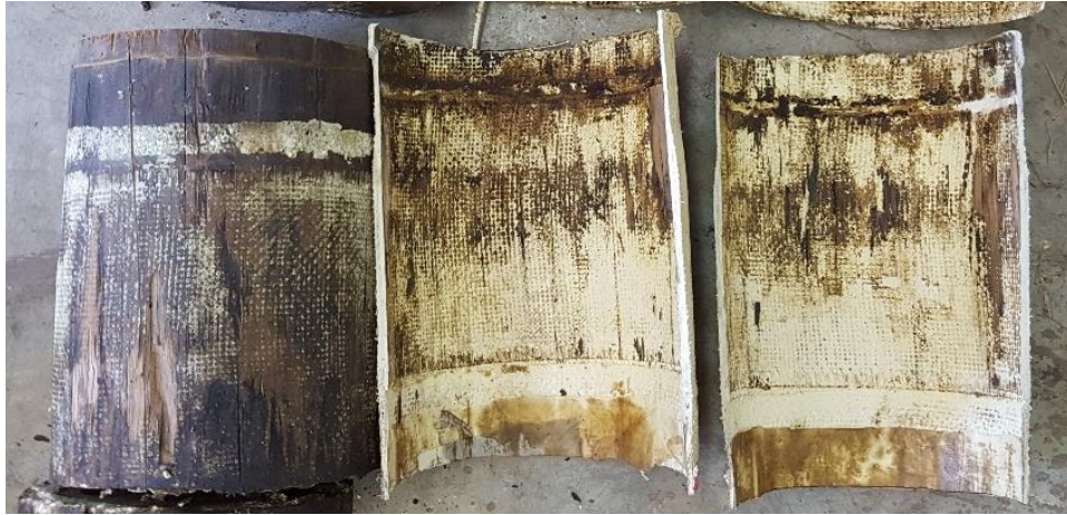
Figure 76. Limited retained timber on Aquawrap 6 in. and 12-in. bond specimens
