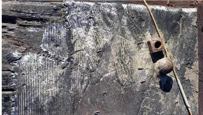
Figure 132. UV degradation of FRP wrap
