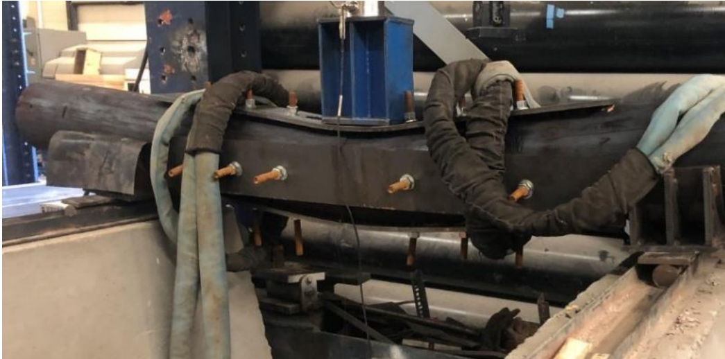
Figure 108. Yielding of top and bottom plates in steel splicing
