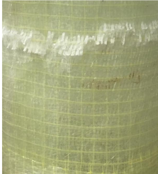
Figure 134. Cracks in FRP wrap
