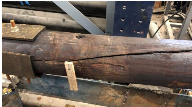
Figure 115. Steel splice cracked pile
