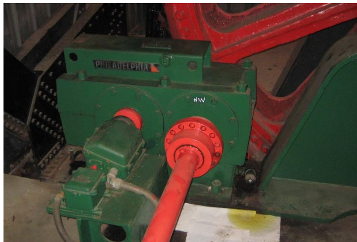
Figure 7. Selsyn equipment outboard of reducer at Bridgeport, CT vertical lift
