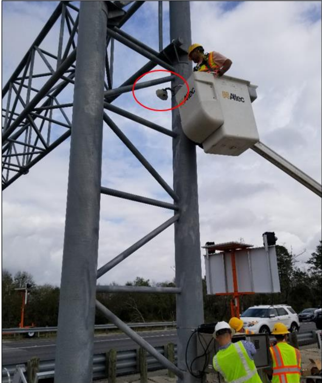
Figure 29. Installation of RTMS device (circled)
