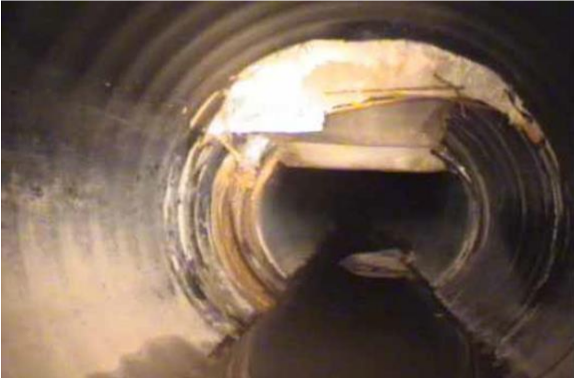
Figure 14. Joint displacement, cracking/fracture, and inverse curvature failures for pipeline in Houston, Site 8 [19]
