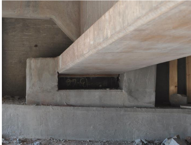
Figure 53. Conditions of the gap between the shear keys and the girder bottom flanges
