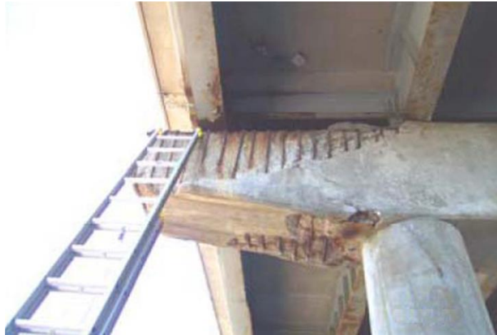
Figure 3. Corrosion damage caused by chloride-contamination leaks in bridge deck expansion joints [6]
