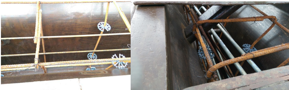
Figure 9: Reinforcement casing inside the form at the Waskey facility in Baton Rouge, LA
