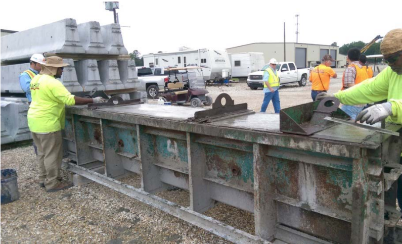
Figure 12: Finishing of the barrier at the Waskey facility in Baton Rouge, LA
