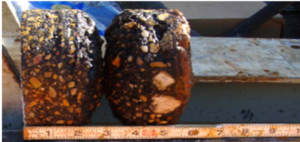
Figure 30 Example of AC stripping in control section 831-06
