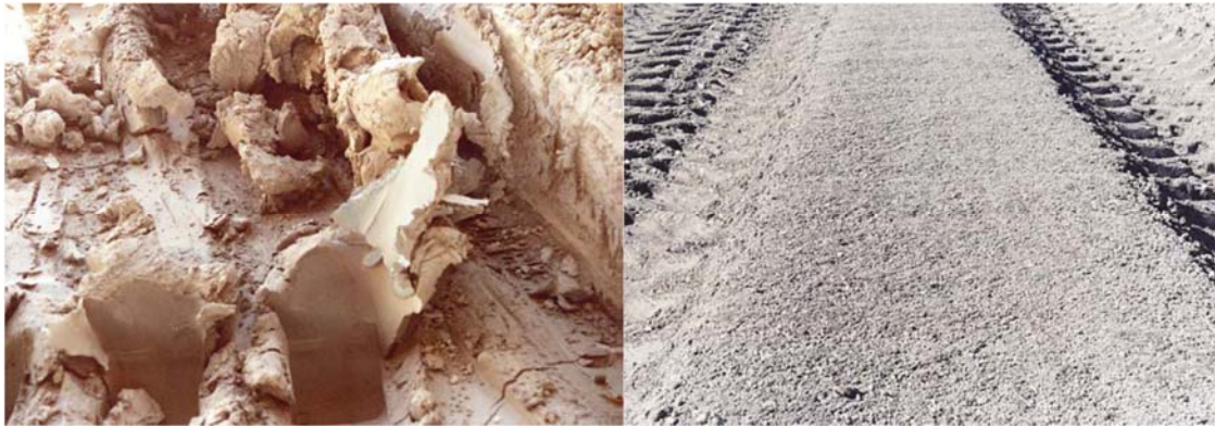
Figure 4 Untreated soft clay subgrade showing highly wet condition (on the left) vs. the same subgrade after lime-stabilization (on the right)
