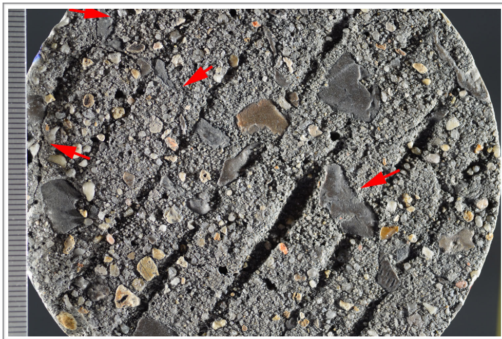
Figure H4. Photographs showing crack (red arrows) on the top surface; scale in millimeters.
