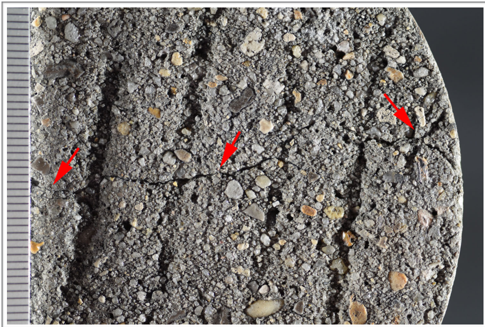
Figure G4. Photographs showing crack (red arrows) on the top surface; scale in millimeters.
