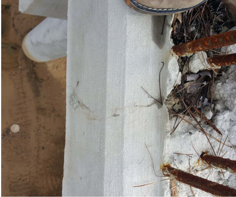
Figure 17 Picture of a mid-span crack on end of the U.S. 80 bridge deck
