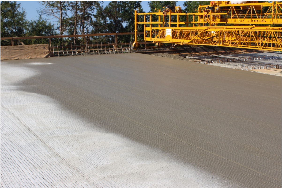
Figure 19 150 pcy ICC placement, note the lack of curing compound in the right of the picture
