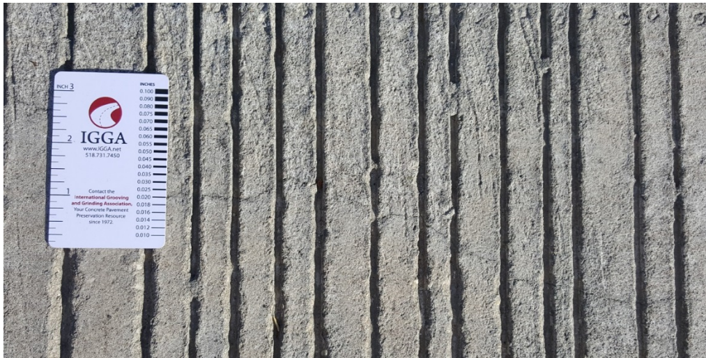
Figure 11 West Congress control span crack size
