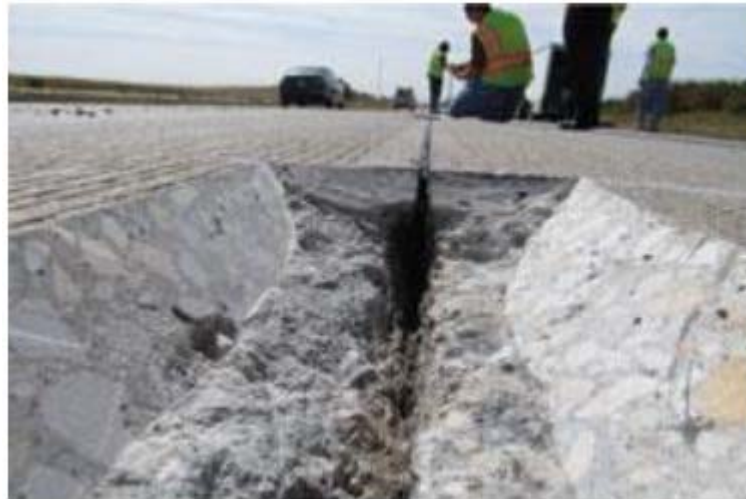
Figure 3 Example of pavement joint deterioration [15]
