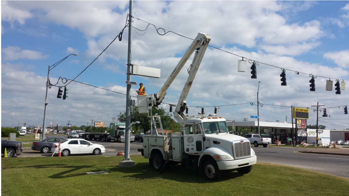
Figure 25 Installation of Bluetooth probe detection system
