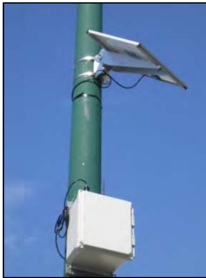
Figure 3 Bluetooth device mounted on a light pole
