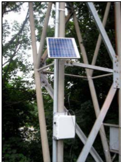
Figure 4 Bluetooth device mounted on a truss
