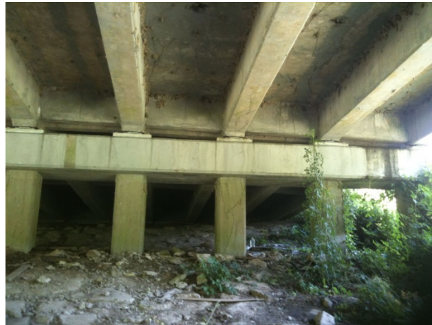
Figure 29 Overall view: Note the debris buildup on the un-coated right side of the structure
