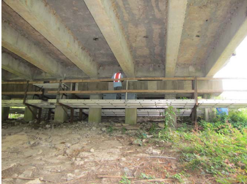
Figure 13 Appearance of the pier cap after initial major repair
