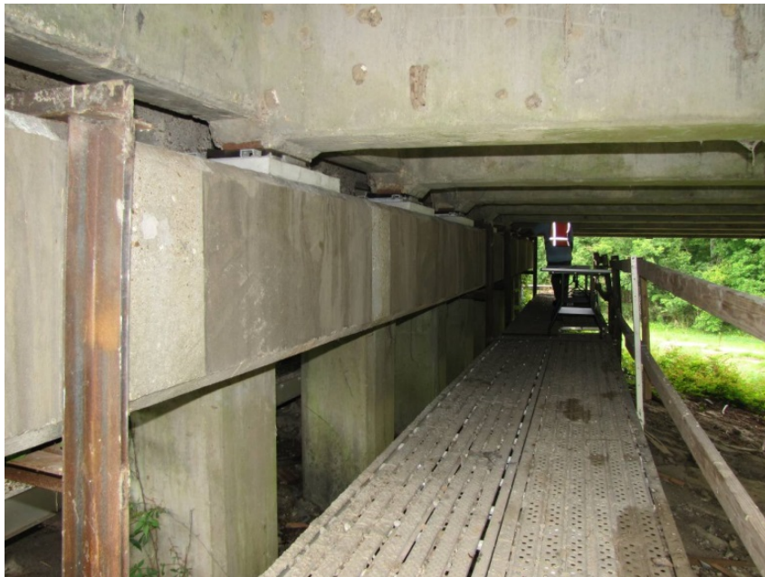
Figure 14 Surface after cleaning with water
