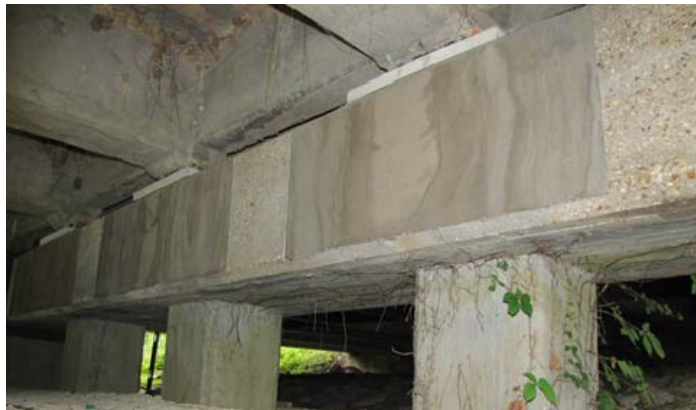
Figure 2 View of the bent after the initial repair: Note the base plates under the beams and the repair material that replaced delaminated concrete
