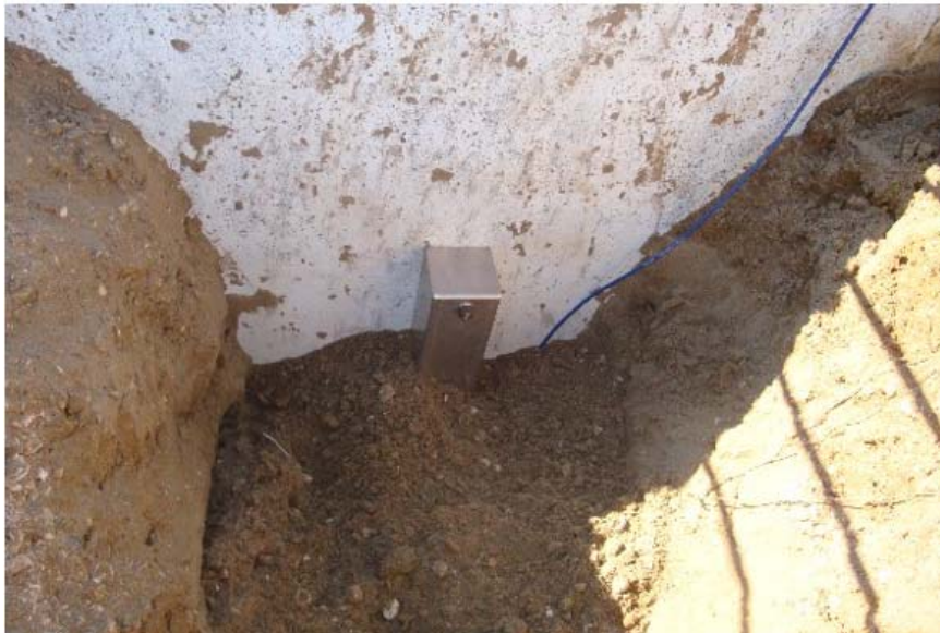
Figure 13 Tiltmeter mounted on Bent 1 face
