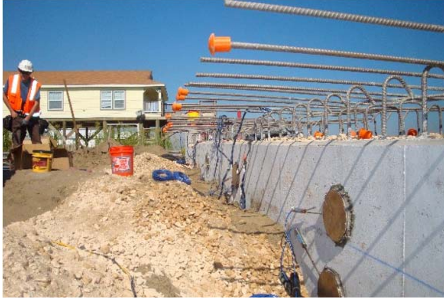
Figure 12 Pressure cells mounted on Bent 1 face
