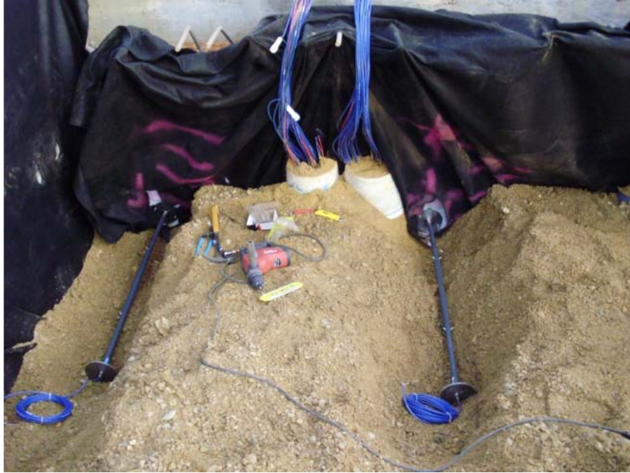
Figure 26 Installation of deformation meters on the back face of Bent 1 of Bodcau Bayou Bridge
