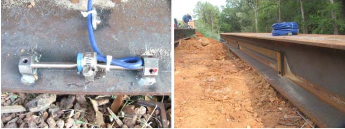
Figure 22 Photo of strain gage welded on the pile flange and cover plates to protect wiring
