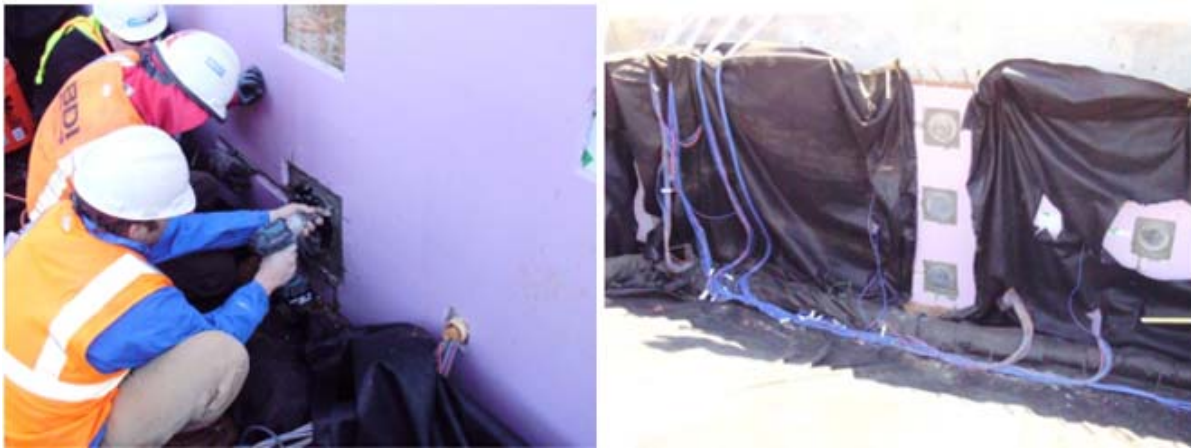
Figure 25 Installation of four pressure cells on the back face of Bent 1 of Bodcau Bayou Bridge
