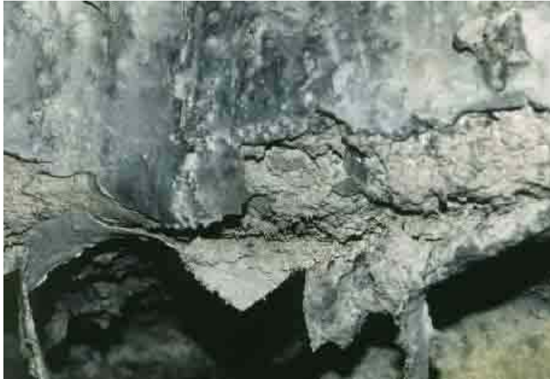
Figure 3 Acid producing bacteria penetrating and colonizing concrete [18]
