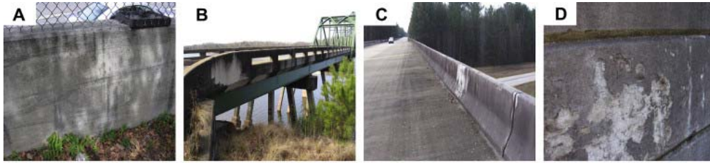
Figure 4 Concrete damage caused by fungi [19]
