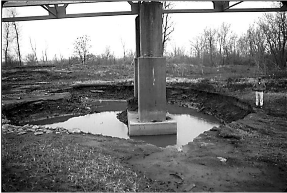
Figure 21 A picture showing the local scour around a bridge pier
