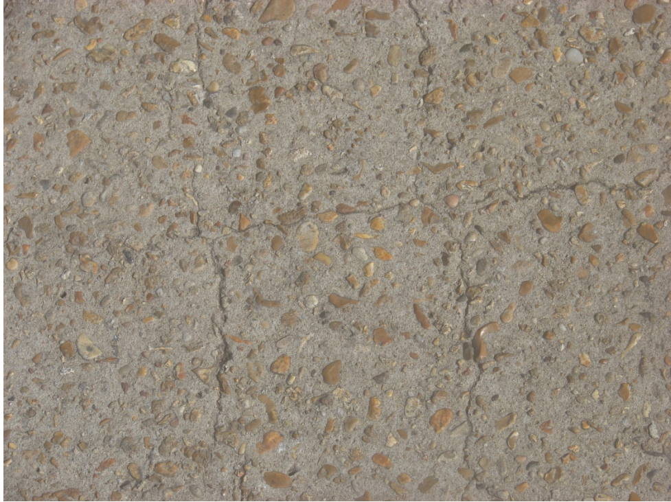
Figure 2 Exposed aggregate and crack pattern (Note the crack pattern is approximately 4 – 6 inches square)
