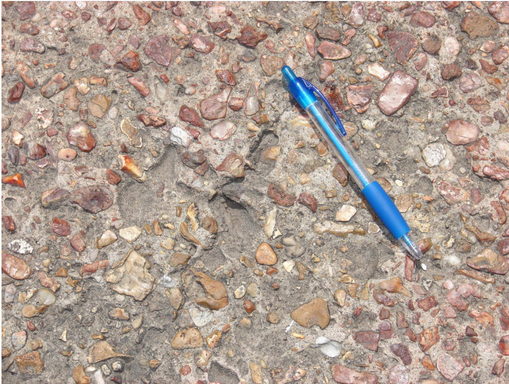
Figure 4 Surface texture and color in span 105 southbound, a fire affected span
