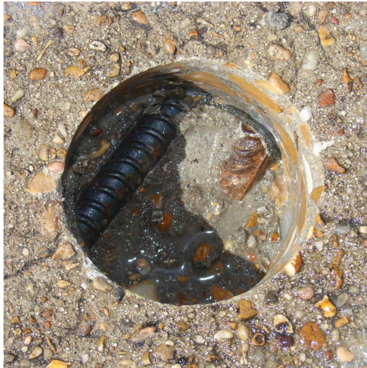
Figure 6 Partial depth core showing little steel corrosion
