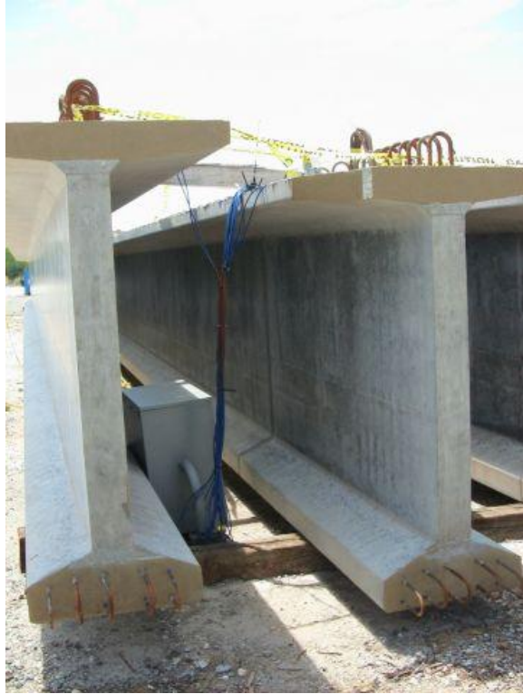
Figure 53 Datalogger location while monitoring of curing girders in casting yard
