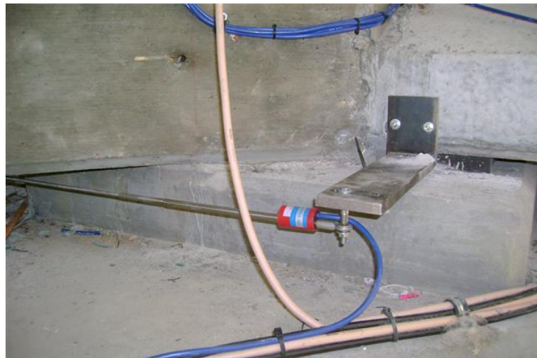
Figure 48 Gap meter installed on brackets connected to girder ends at continuity diaphragm
