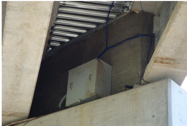
Figure 54 Datalogger location in the complete system at bridge site (Bent 24)
