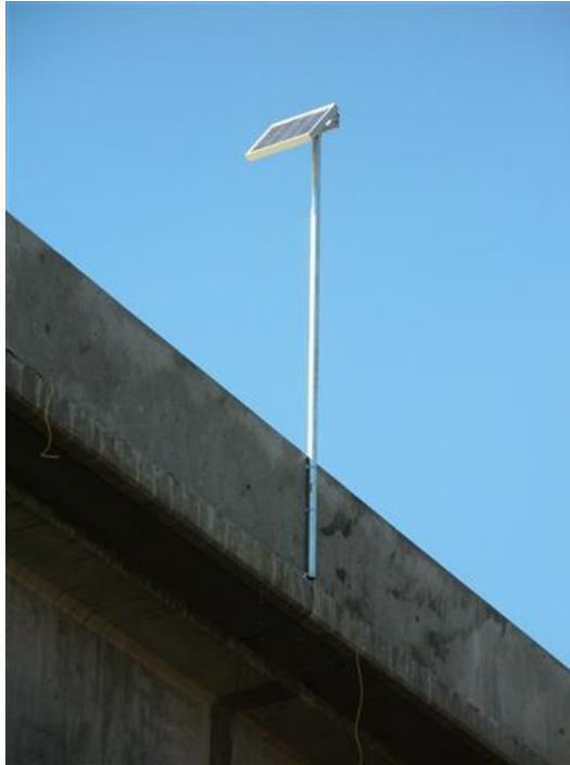
Figure 51 Solar panel powering the monitoring system
