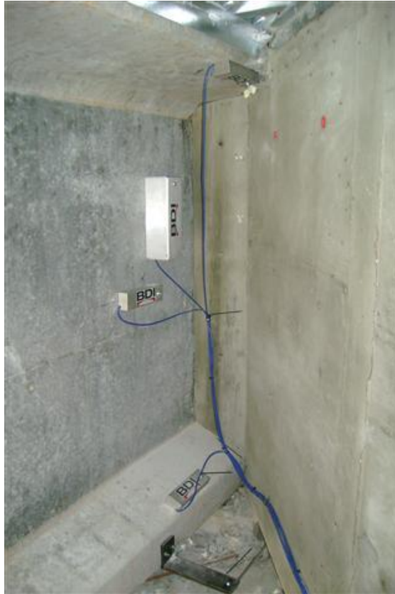
Figure 47 Surface-mounted sensors (vibrating wire gages and tiltmeters) at girder ends
