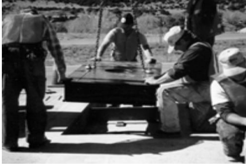
Figure 7 Single load cell installation (source: International Road Dynamics Inc., www.irdinc.com )
