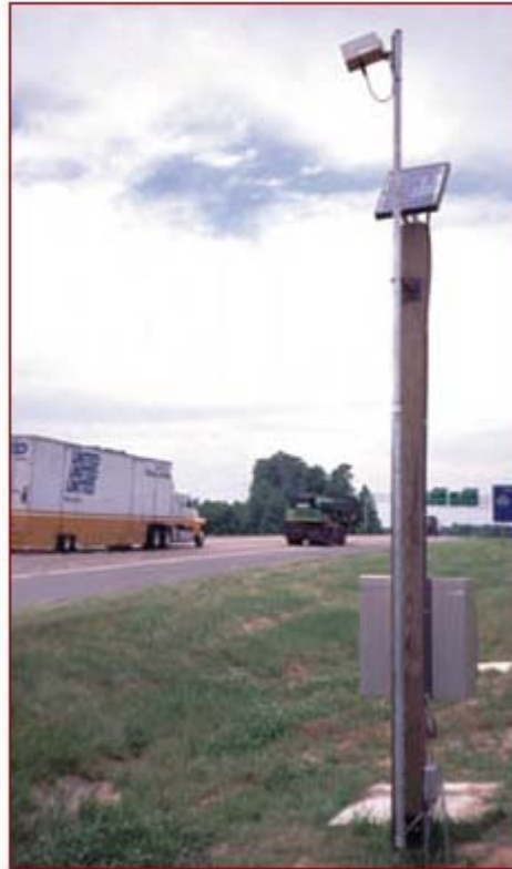
Figure 9 RTMS solar powered remote counting station
