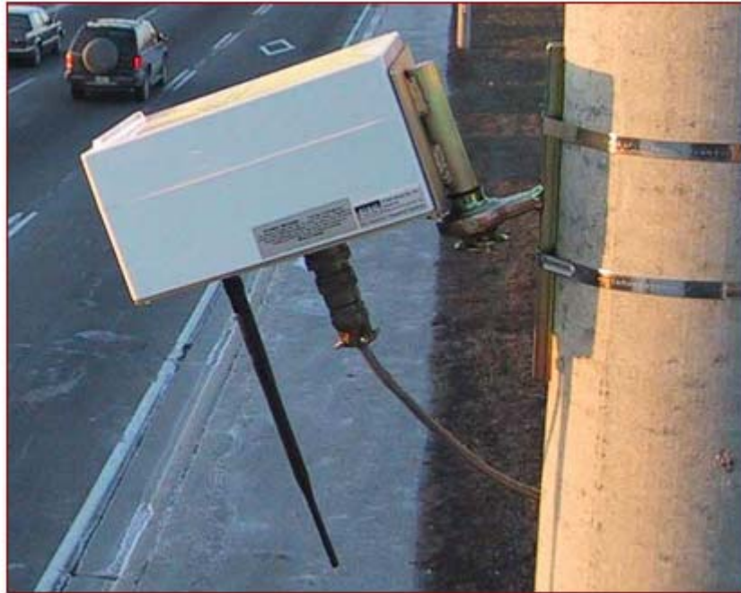
RTMS (Remote Traffic Microwave Sensor) radar
