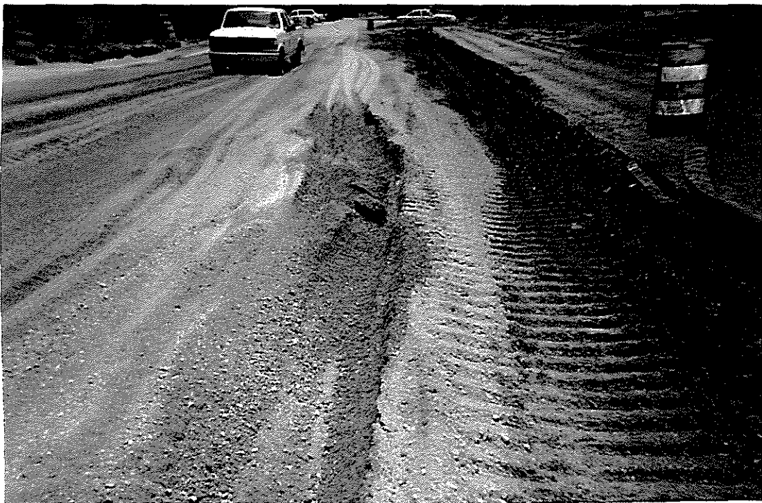
Figure 5 Base course failures
