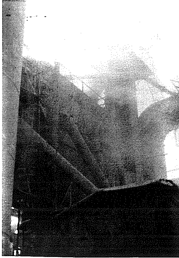
FIGURE 18 DUST LEAKAGE FROM PLANT EQUIPMENT
