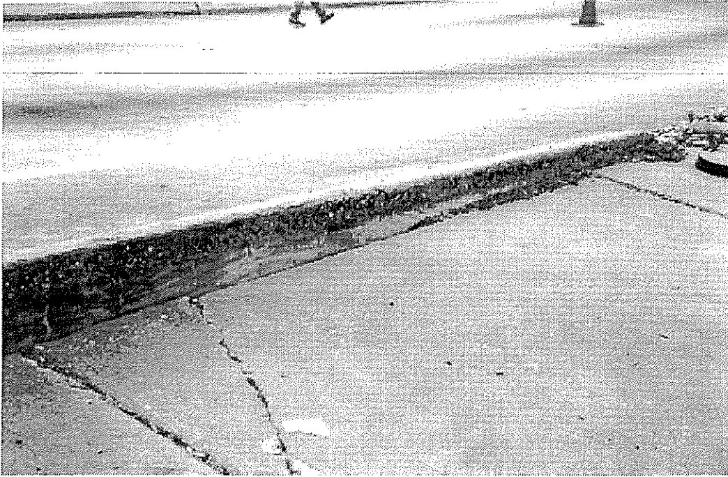
Figure 42 Longitudinal differential settlement between approach slab and its adjacent side shoulder pavement
