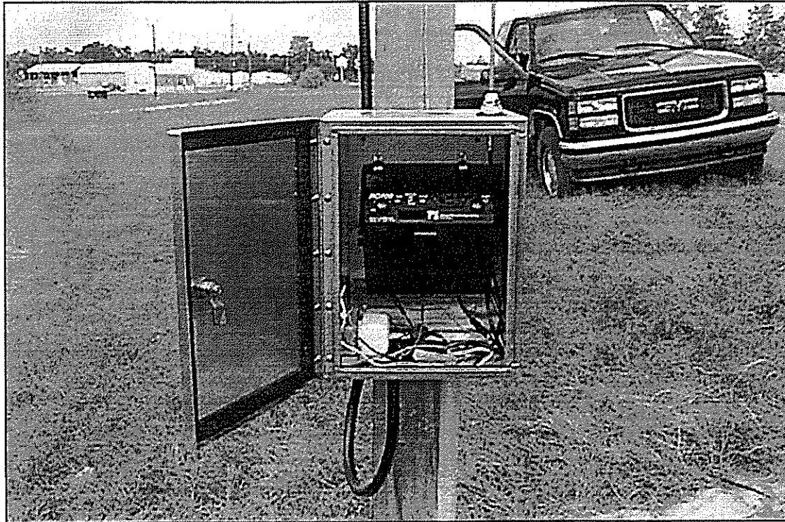
Figure 10 Pole mounted RC 200 flash activation system
