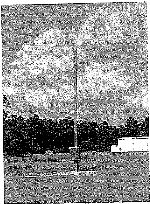
Figure 5 Standard AC powered HAR transmitter station (Moss Bluff, Louisiana)
