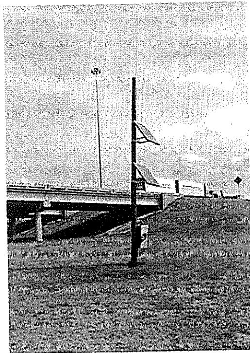
Figure 6 Solar powered HAR transmitter station (located at the I-10/LA 415 interchange, West Baton Bouge Parish)
