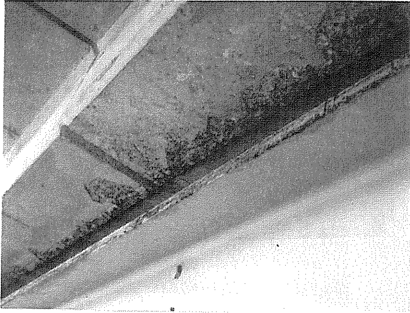
Figure 5 Top flange pulled out of slot
