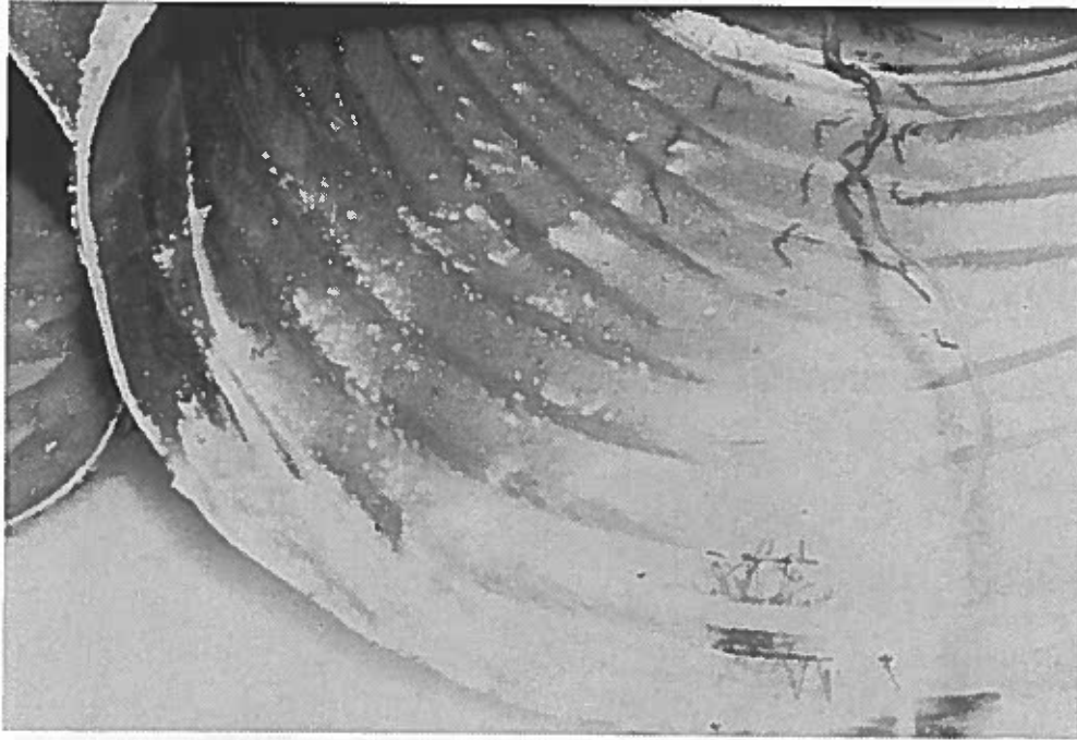
Figure G-9. This is a close-up of the inside of the culvert.
