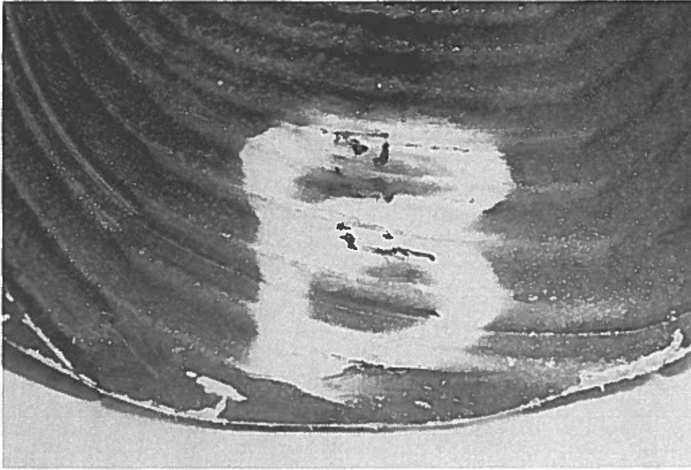
Figure G-26. The inside of this culvert shows a large number of rust spots.
