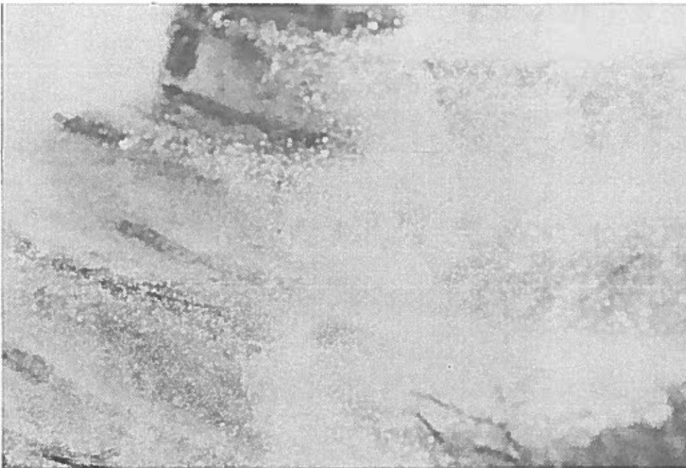
Figure G-27. This is a close-up view of the inside of this culvert which shows corrosion attack.
