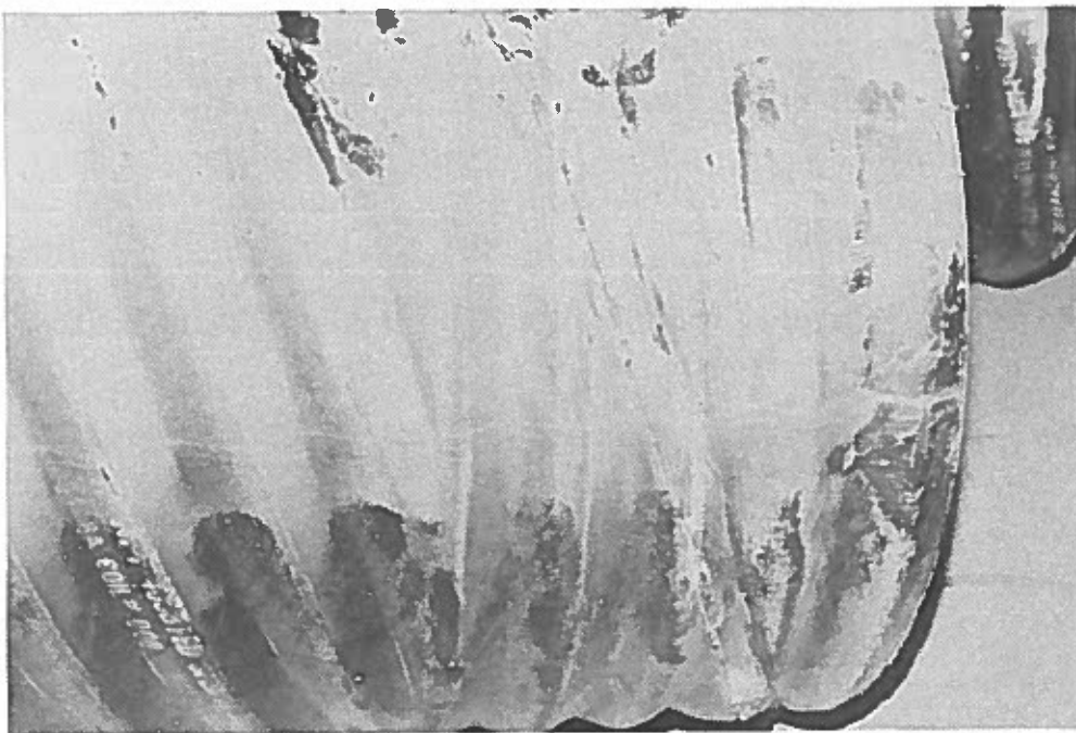
Figure G-15. This view shows very little white powder on the outside of the culvert.
