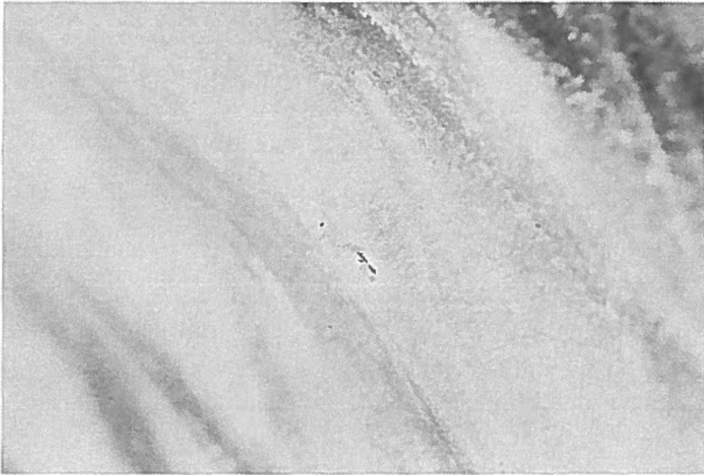
Figure G-30. This photograph shows that external attack has occurred on this culvert.
