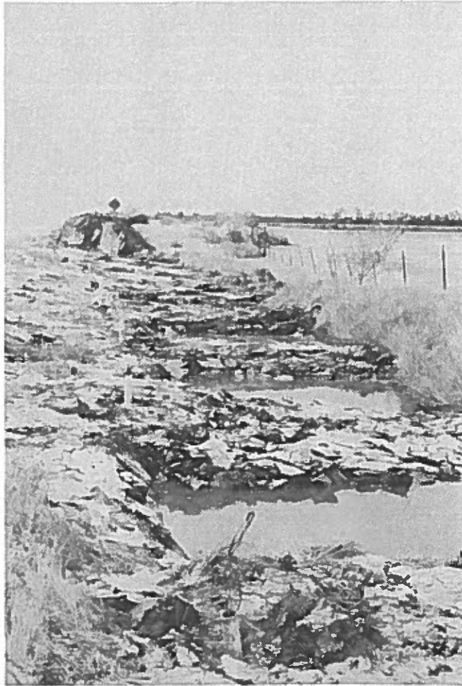
Figure 12. This is what the site looked like after the installation was completed.
