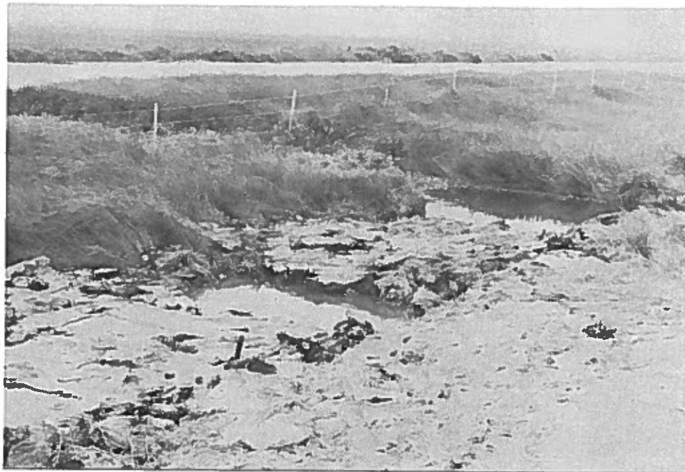
Figure 16. This is what the unprotected site looked like after the installation was completed.
