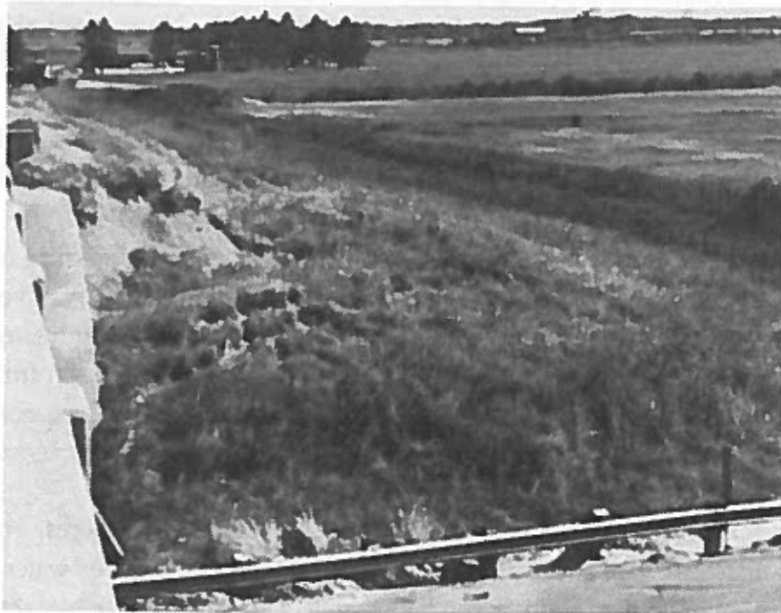
Figure 7. Slump at Locality S15, Acadia Parish, southwest quadrant. Failure morphology is well displayed: head scarp, rotated inward slump blocks, and toe above the guard rail.
