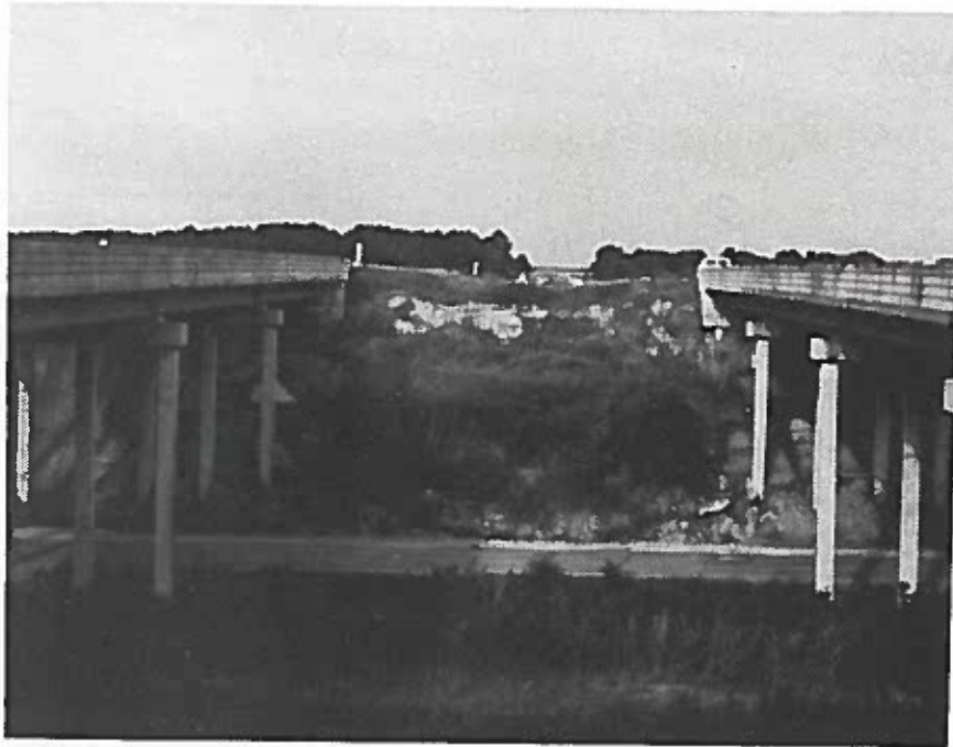
Figure 16. Slump failure between two bridges on I-10 (Locality S12, AC-Bridge, east side). Note the broken and displaced sections of concrete revetment apron.
