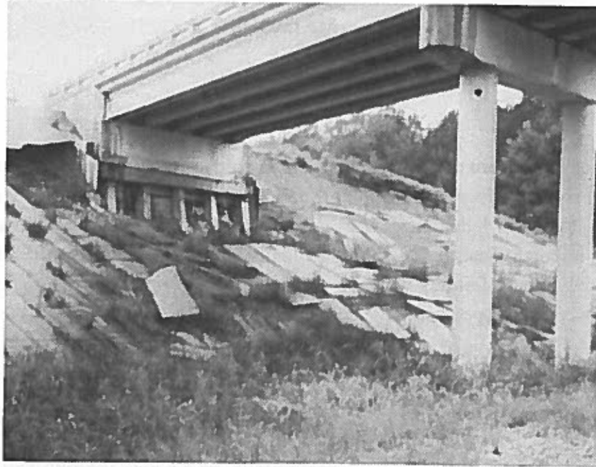
Figure 6. Slump at Locality S12, Acadia Parish, east side of overpass. The slump is 32 m wide and 21 m long. Scarp is 2.5 m high. Note the displaced sections of concrete apron.
