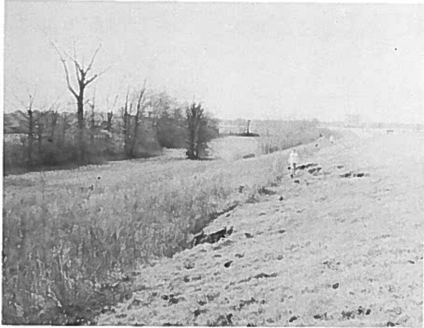
Figure 13. Slump-earthflow at Chicago Mill, southwest quadrant, Locality N17, Madison Parish, I-20 study area. The high vegetation masks the failure. This failure continued to grow throughout the duration of the study.
