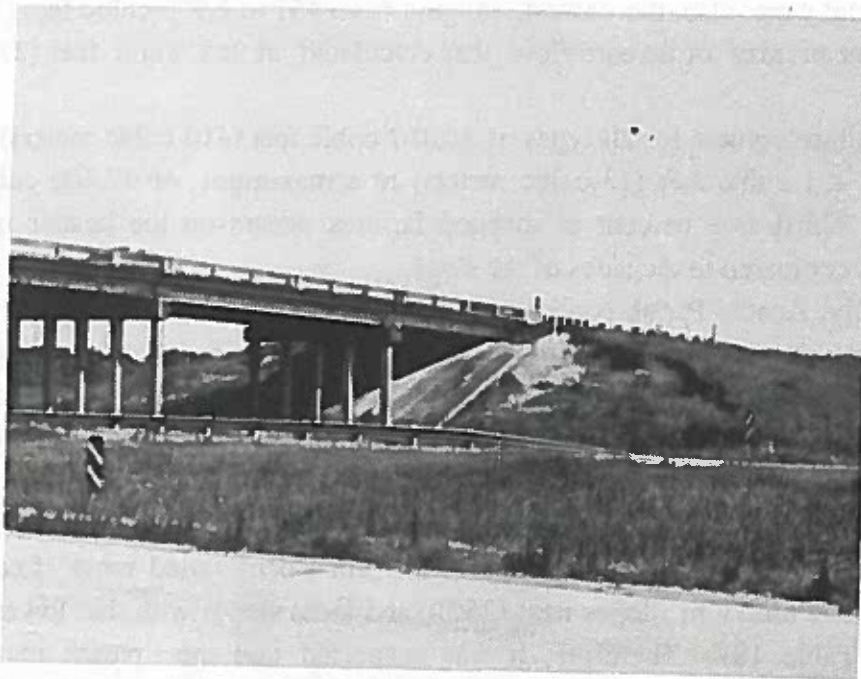
Figure 17. Slump-earthflow beginning to undermine the revetment apron at Locality S15, AC-EO1111-SW.
