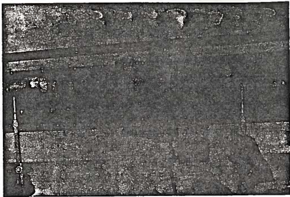
Figure 54. Line Heat Applied to the Yield Line of the Web of Girder SB-2
