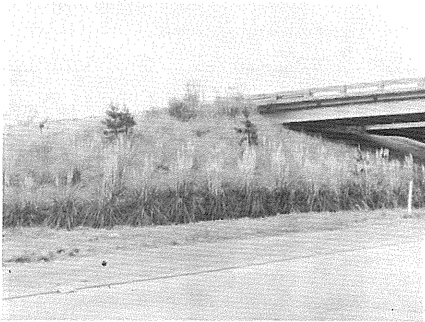
Figure 10. Slope stabilization with exotic vegetation. At this locality S1 in Calcasieu Parish in the I-10 study area, pampas grass has been successfully used to stabilize a repaired slope.
