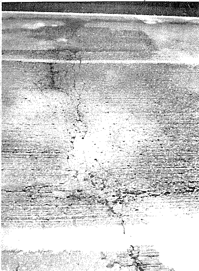
Rough Concrete Test Section on La. 2 in North Louisiana. Actually a Thin Asphalt Overlay Covering an Old Concrete Slab.
