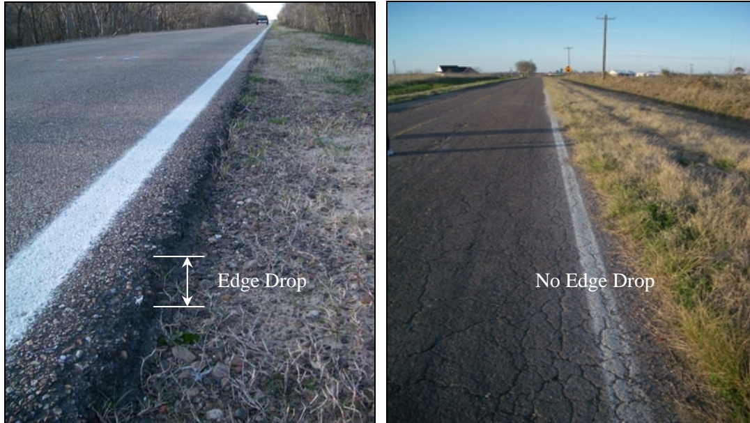
Figure 32 Pavement edge drop
