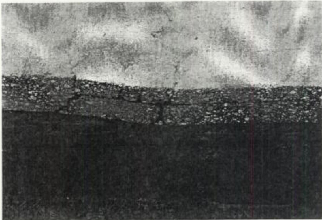
Figure 23 Post-mortem of lane 006
