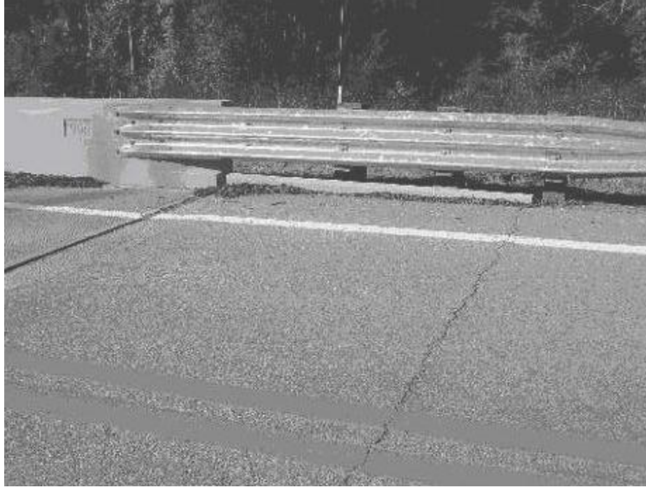
Figure 18 A crack across the approach slab of Bridge C-1
